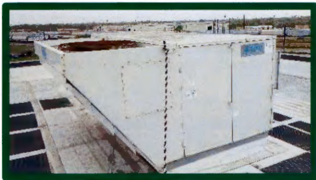
Aging/failing Roof Top unit at the Police Station
