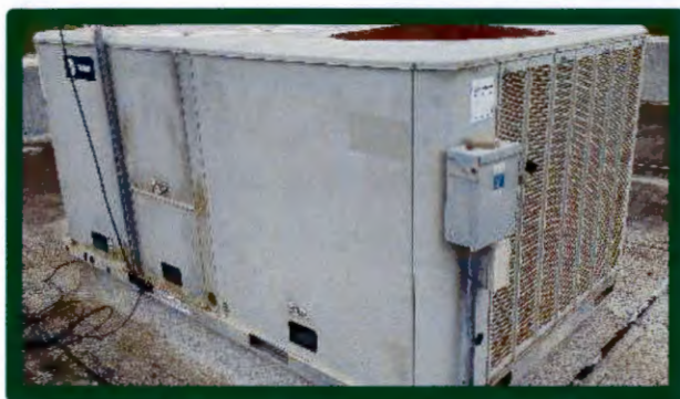
Roof Top Unit at City Hall from 2004
