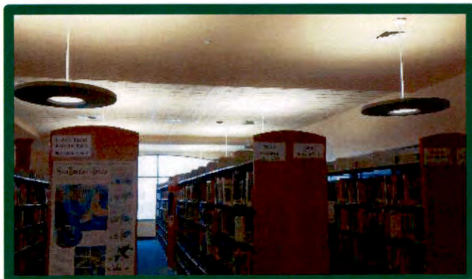
Library inefficient fluorescent lighting
