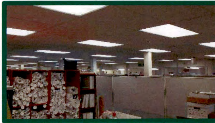
Lon C Hill inefficient fluorescent lighting
