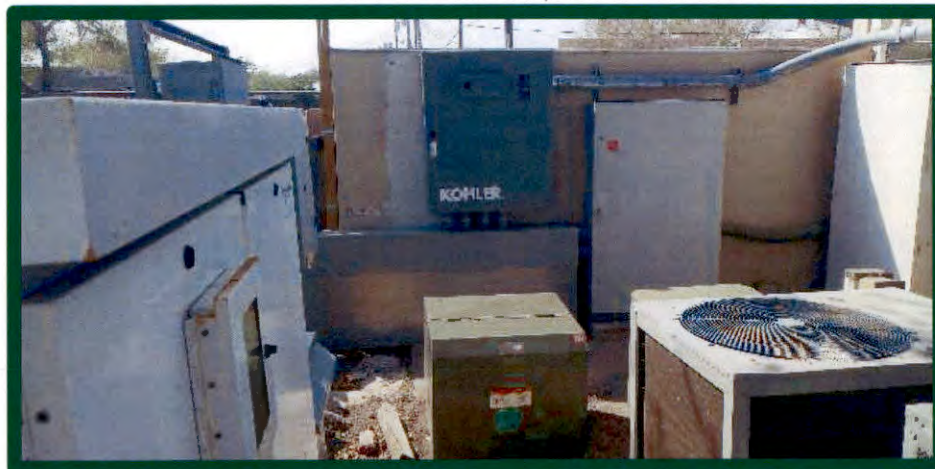
Inverter and electric panels for the Solar PV at Lon C Hill
