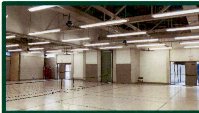
Harlingen Community Center inefficient fluorescent lighting
