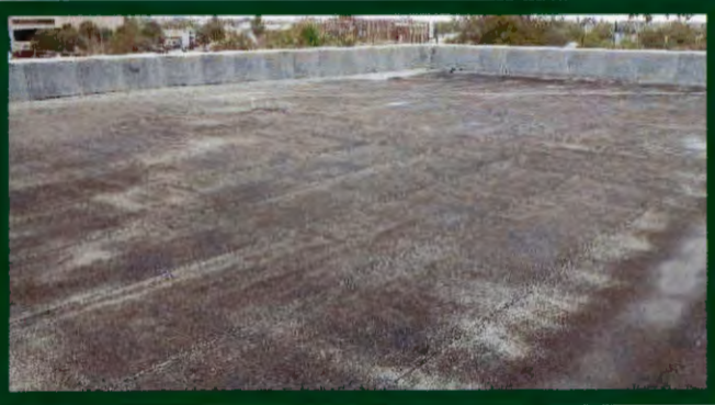
City Hall roof at or past expected service life
