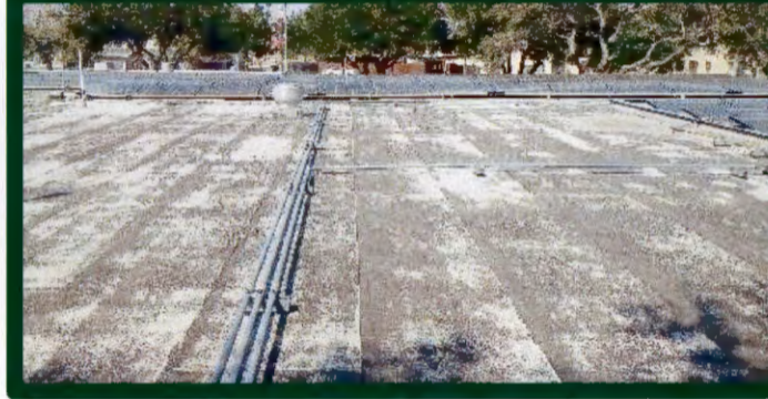
Lon C Hill roof at or past expected service life
