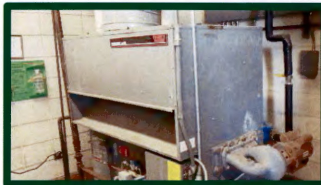
Aging/failing boiler at the Community Center
