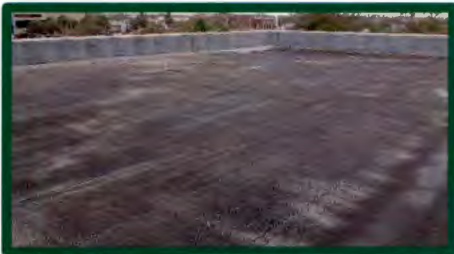
City Hall roof at or past expected service life
