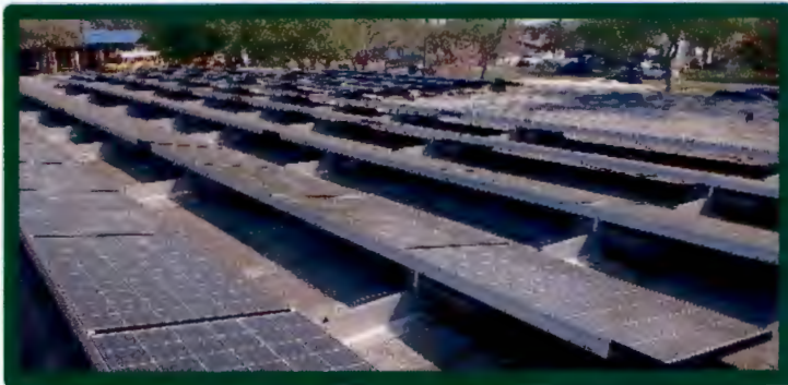
Solar Photo Voltaic Panels at Lon C Hill
