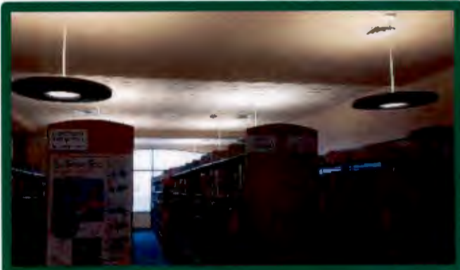
Library inefficient fluorescent lighting
