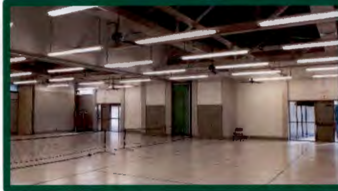
Harlingen Community Center inefficient fluorescent lighting
