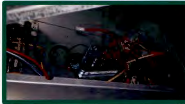
Problematic VAV box at the Police Station
