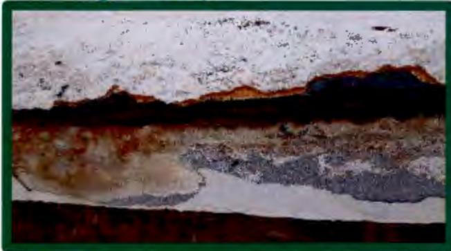
Casa Del Sol roof edge in need of Repair
