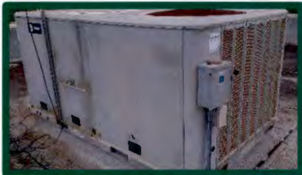
Roof Top Unit at City Hall from 2004
