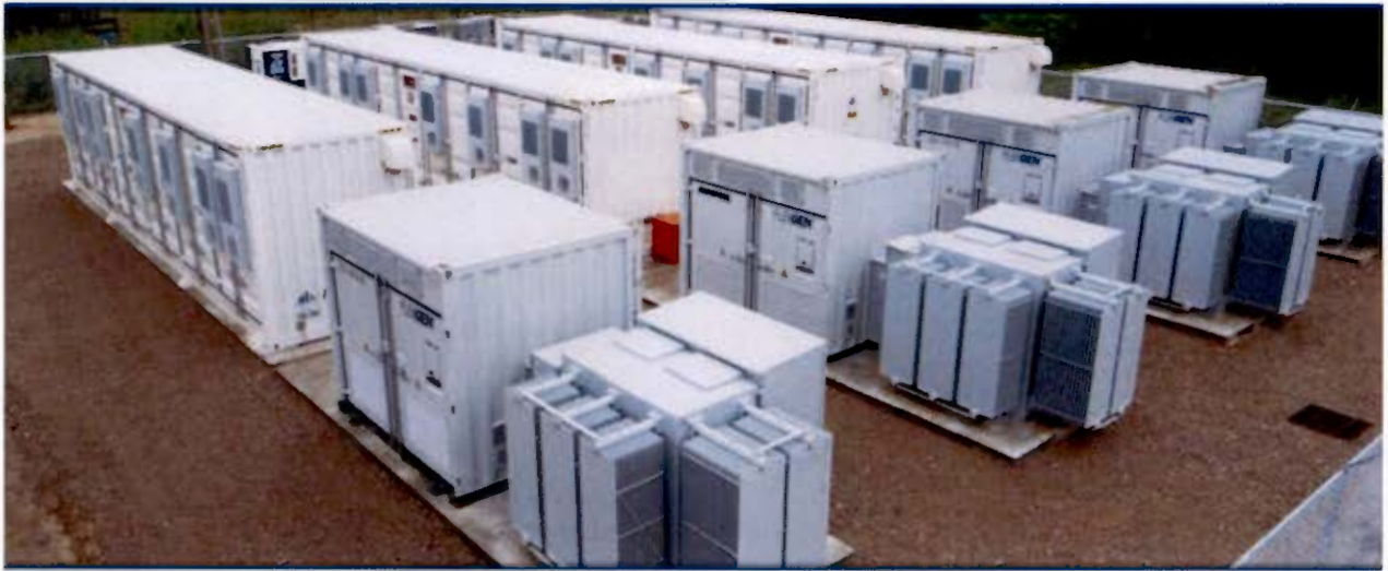
Example of a battery storage energy facility
